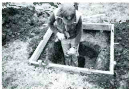
The hole for the pad was slightly deeper than 3ft at the deepest point. Note the terracing of the hole.
