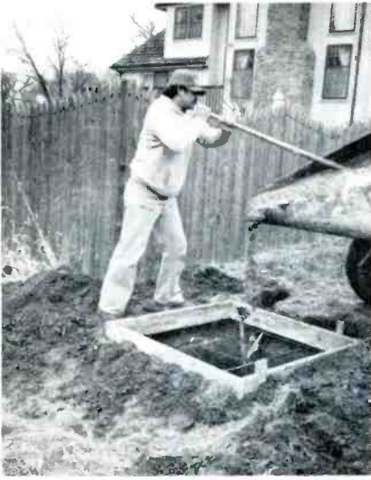
The concrete is poured, leveled and allowed to set for at least two days.
